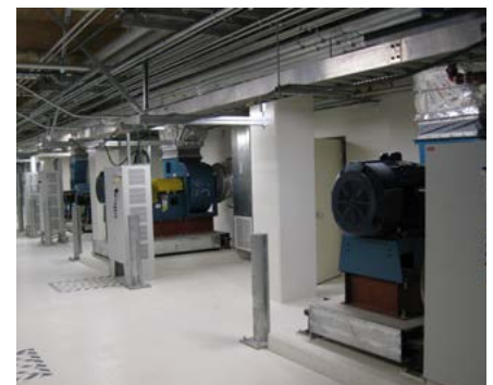
Exhaust Fans for Nuclear Plant
