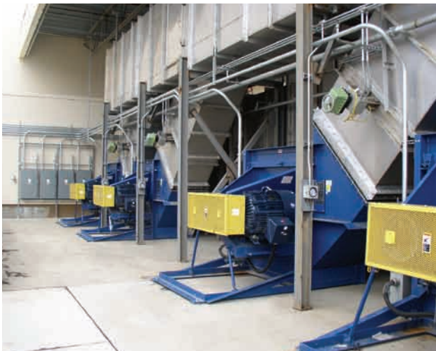
Swingout fans in a paint booth application
